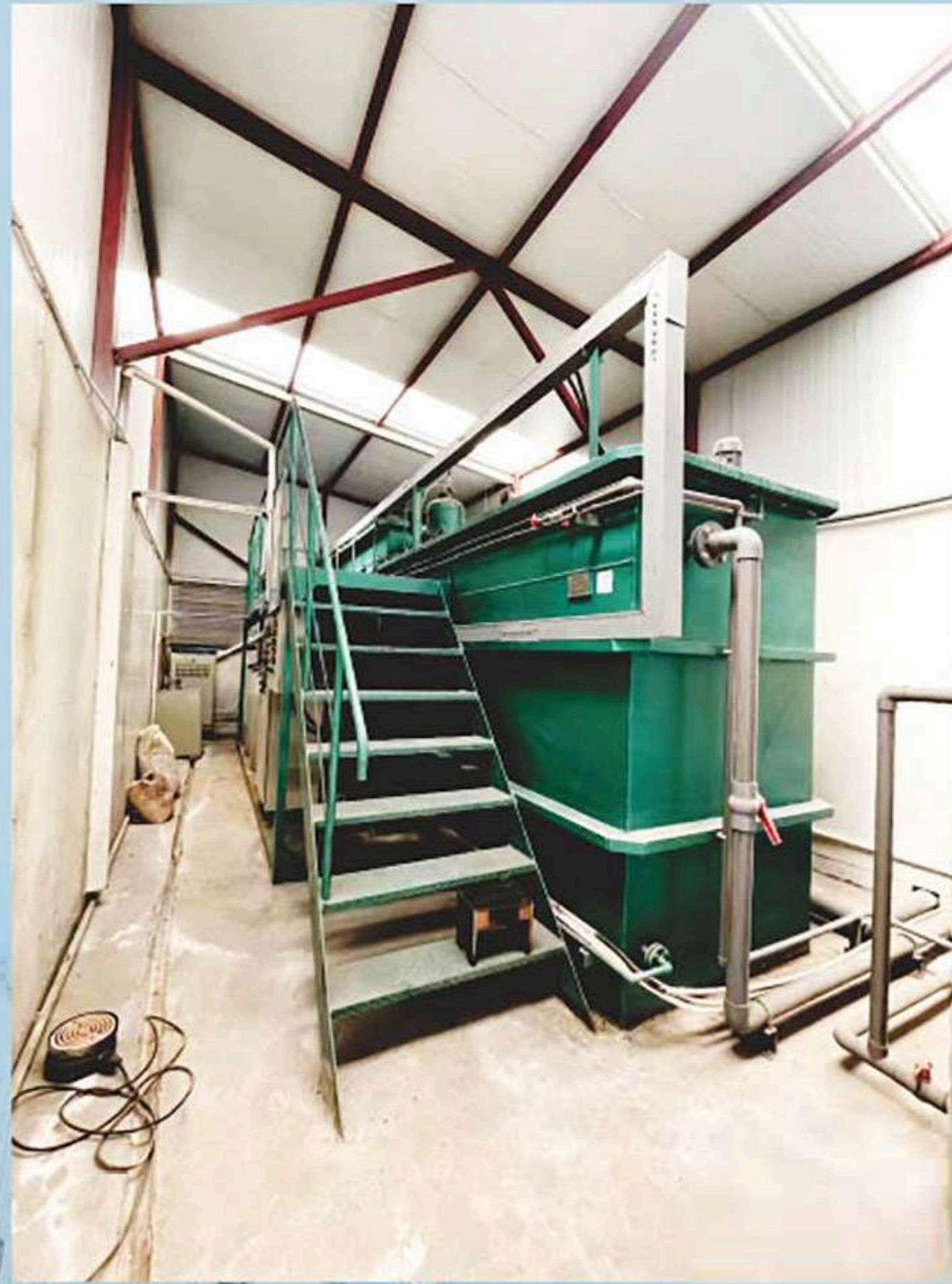
Environmental Protection Facilities
